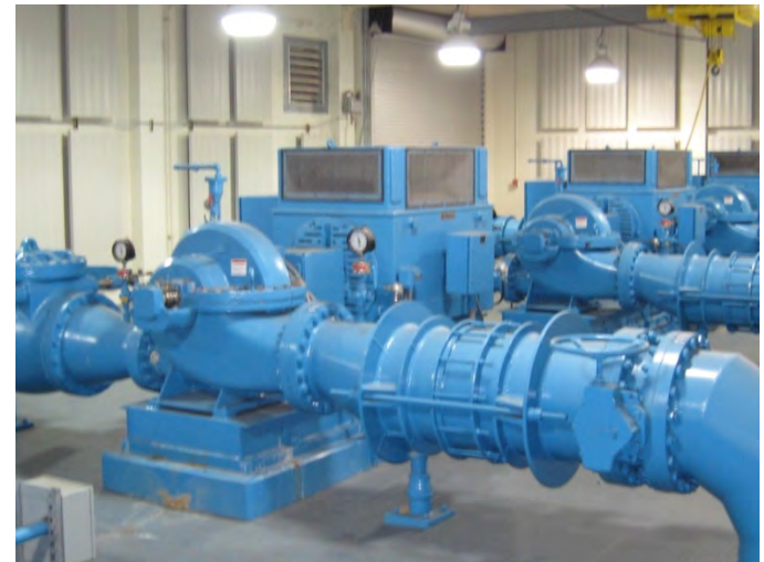
Hesperian Pump Station
