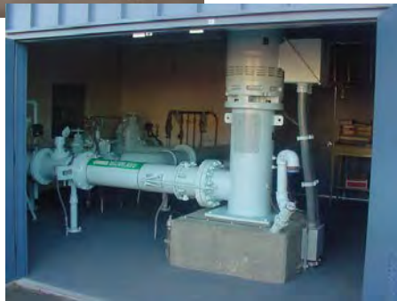
Emergency Well and Pump
